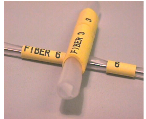
PO-MARKERS ON OPTIC CABLES
